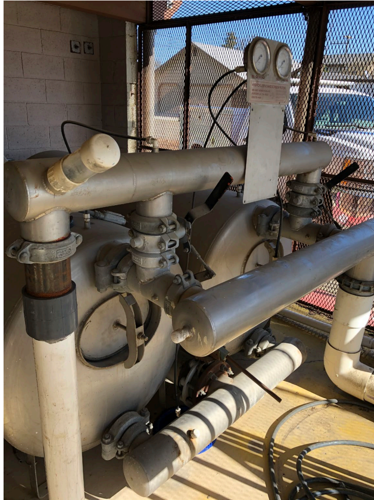
Swimming Pool Filter Tank System
